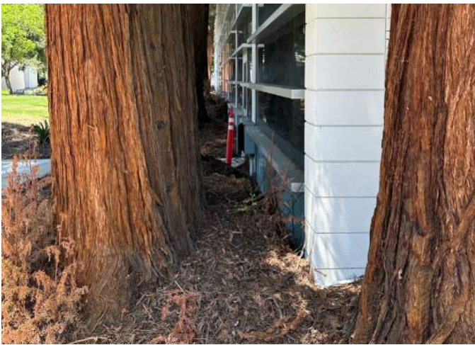
Photo: The redwood trees around the Business Building are encroaching on its foundation.
