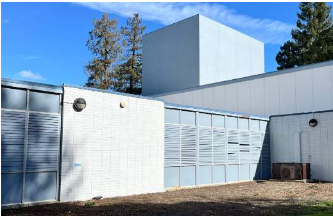
Photo: The Theater Arts/Drama building is not in good condition. It was identified for removal in the last FMP Update.
