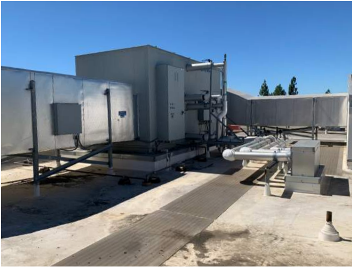
Photo: The Central Plant at EVC is being replaced, and could be made all-electric in the process.
