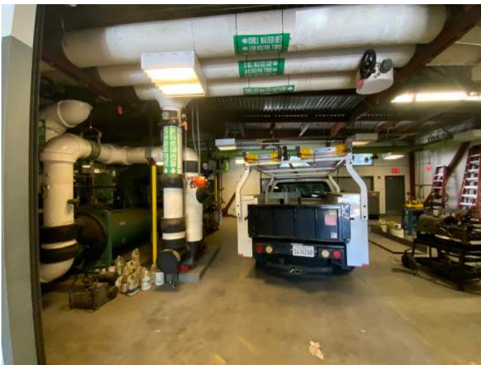
Photo: SJCC Central Plant
