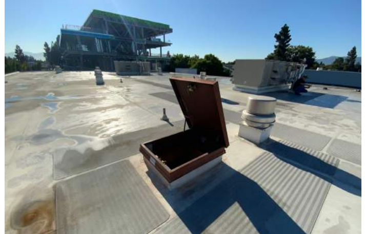
Photo: The roof access hatch curb has not been painted on most buildings. The base paint is red oxide and gets very hot during the summer.
