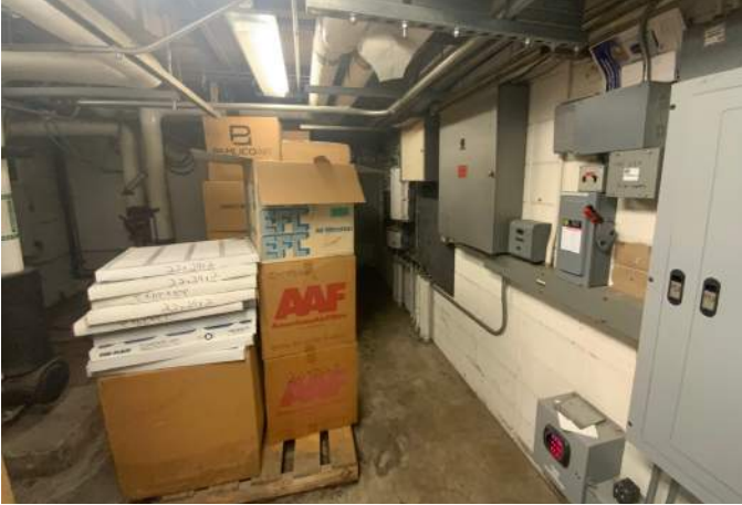
Photo: Several Mechanical Rooms are used for storage. This could be hazardous for the facilities engineers.
